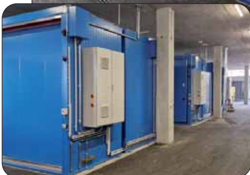
◆ Fire protection containers were integrated in the building complex (first floor)
