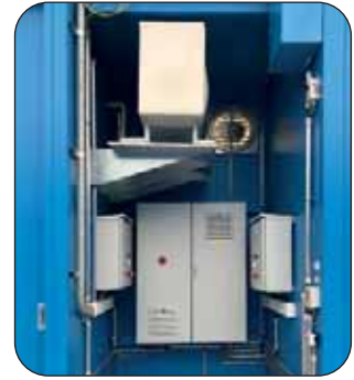
◆ Central control unit (control cabinet, sub-distribution, cooling unit)
